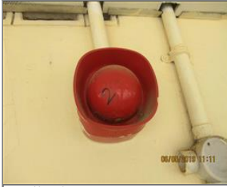
Photo of fire safety equipment Fire alarm.jpg
